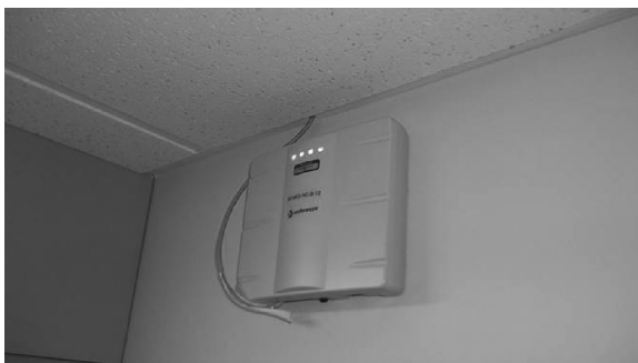
Figure 9.3 Example of poor cable installation.
